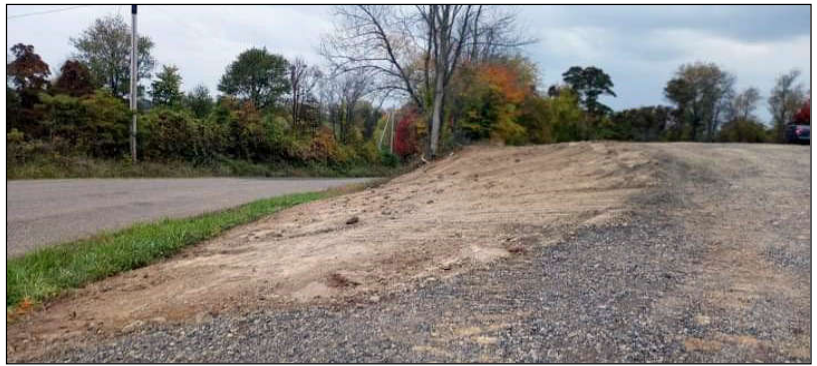
A contractor was recently hired to remove the blind spots on either side of the road at the entrance to The Preserve Trailhead as further development of this project continues.
