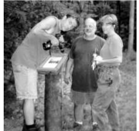
With his parents looking on, Nick Zorko (left) installs the last of 42 new signs along the Heritage Trail.
