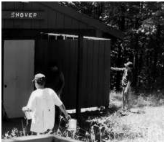
Mark Starchan of Troop 122 rebuilt the shower stall area at the showerhouse. Troop 301 (above) painted the showerhouse inside and out.
