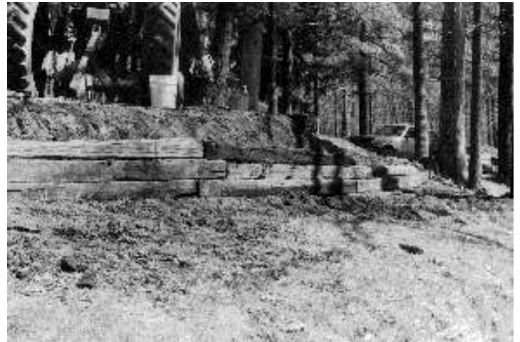
Mike Seaburn of Troop 144 removed and replaced a railroad tie wall on the south side of Kimble Hall.
