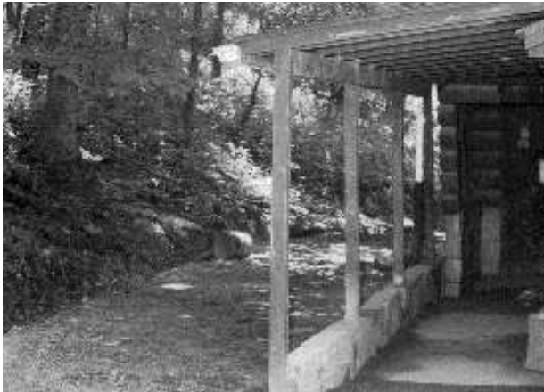
Joe Butts of Troop 25 repaired the porch supports at Jamboree Lodge, regraded the area for drainage and installed drain pipe. Trustee Bernie Richard assisted.
