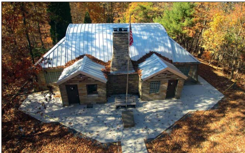
Hoover Lodge sports a new metal roof, new windows, new doors, new cement walkways and a freshly-cleaned exterior. Watch for updates on the interior work that is now under way.
